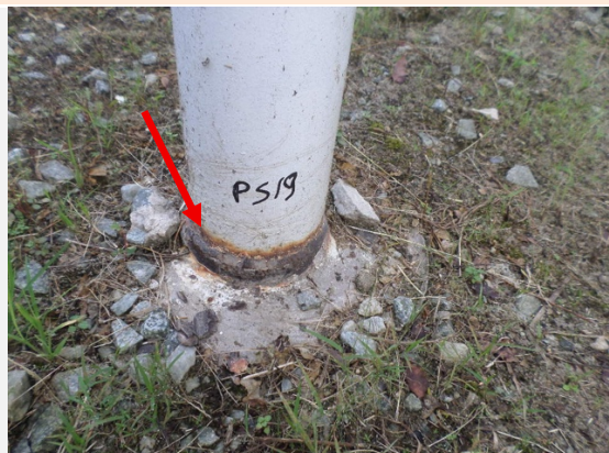
Photo: 5 Comment: Pipe support foundation, at PS19 found with corrosion at the foundation.
