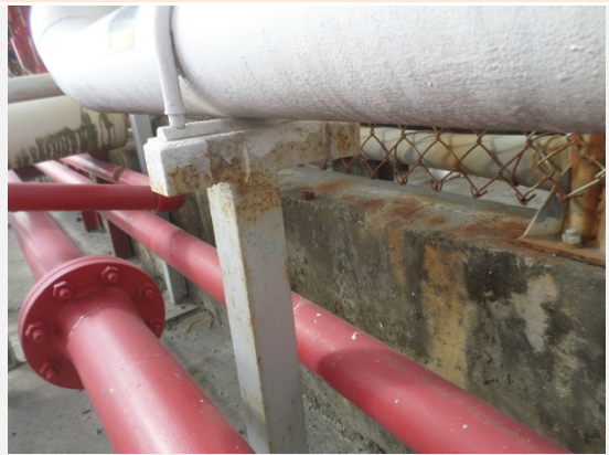
Photo: 10 Comment: PS56 – Coating breakdown and surface corrosion on the beam support
