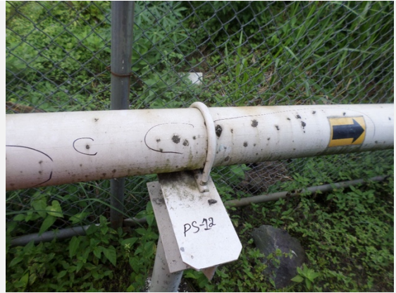
Photo: 14 Comment: Localized concrete spatter located downstream and upstream of pipe support PS12.
