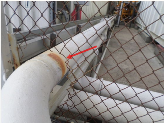
Photo: 35 Comment: Staining, from the metal fencing, noted at the location no 176. No damage to coating noted yet.
