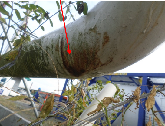
Photo:3 Comment: Elbow component, location 8 on iso, found with localized corrosion
