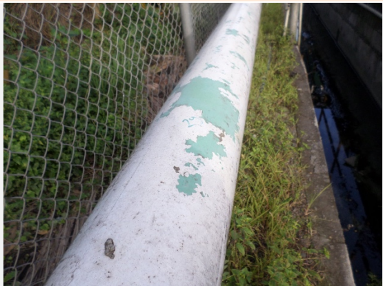
Photo: 9 Comment: Topcoat damage to the section of the line, location: between pipe supports PS9 and PS10
