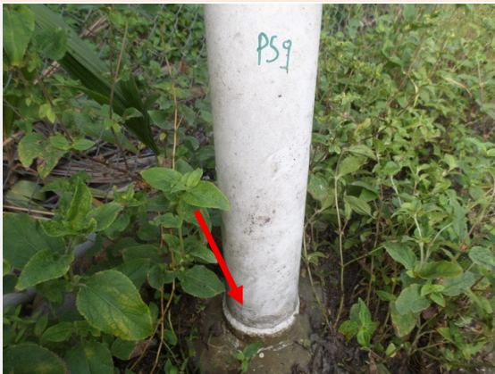
Photo: 3 Comment: Pipe support foundation, at PS9 found with surface corrosion at the foundation.
