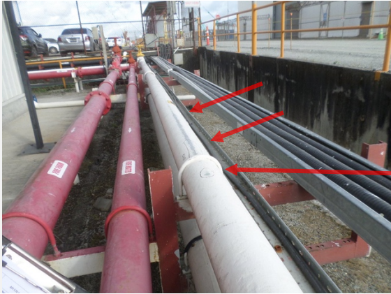
Photo: 31 Comment: Isolated minor coating breakdowns on the line, location: around pipe support PS40
