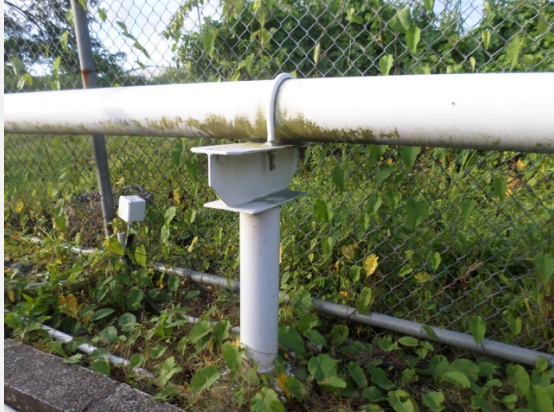
Photo: 1 Comment: Pipe support PS3 – typical condition, generally good, of the supports (except for the supports reported below) on the line.
