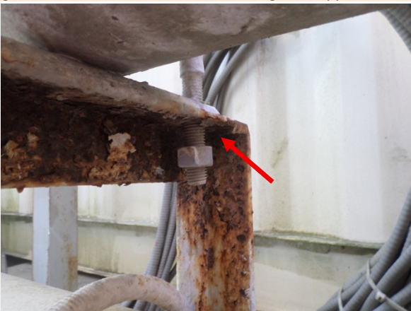
Photo: 17 Comment: PS59 – U-bolt fastener not tightened, stuck in the position, possible thread damage
