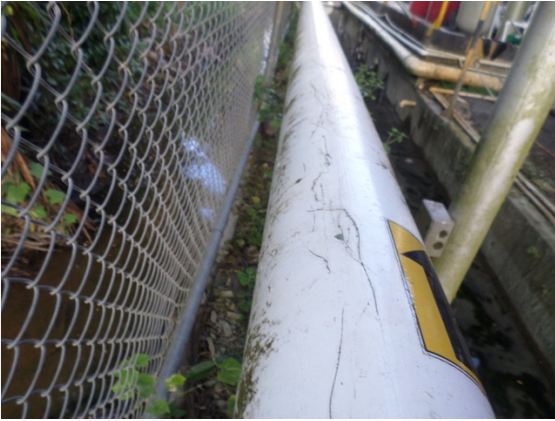
Photo: 7 Comment: Localized, minor, mechanical coating damage located at 12 o'clock, between pipe supports PS6 and PS7.
