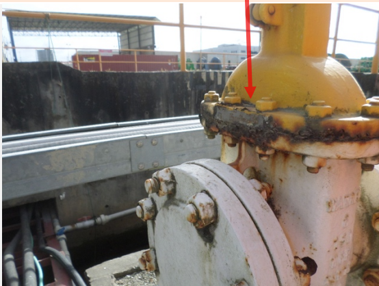
Photo: 29 Comment: Close-up photo Crevice corrosion noted on the bonnet to body, flanged joint. Valve upstream of T-Piece.
