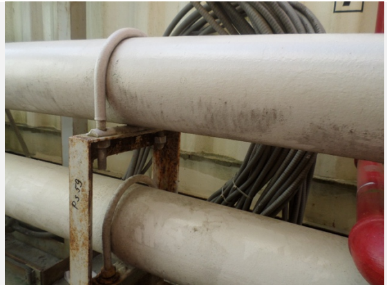
Photo: 16 Comment: PS59 - Coating breakdown and surface corrosion on the support
