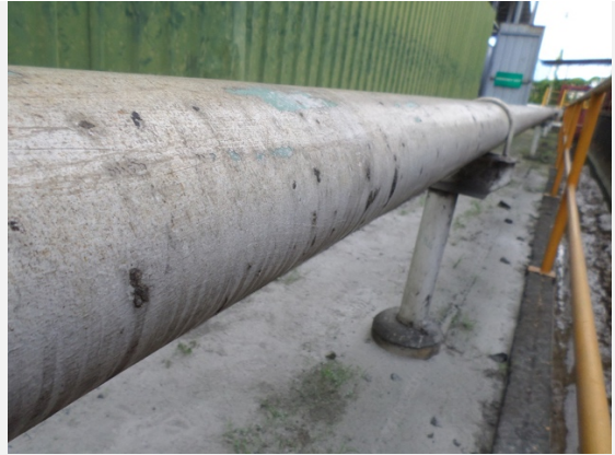
Photo: 20 Comment: Isolated concrete spatter noted at the line, location: between pipe supports PS26 and PS27
