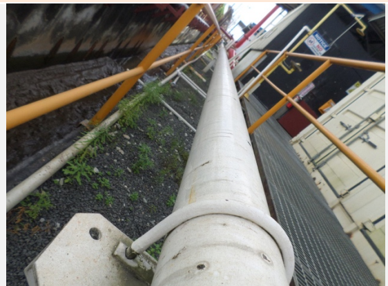
Photo: 22 Comment: Isolated, minor concrete spatter noted at the long span of the line, location: between pipe supports PS29 and PS32
