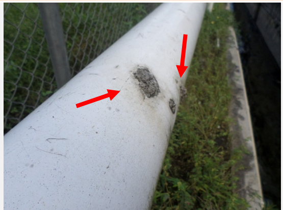
Photo: 11 Comment: Isolated concrete spatter noted at the line, location: between pipe supports PS10 and PS11
