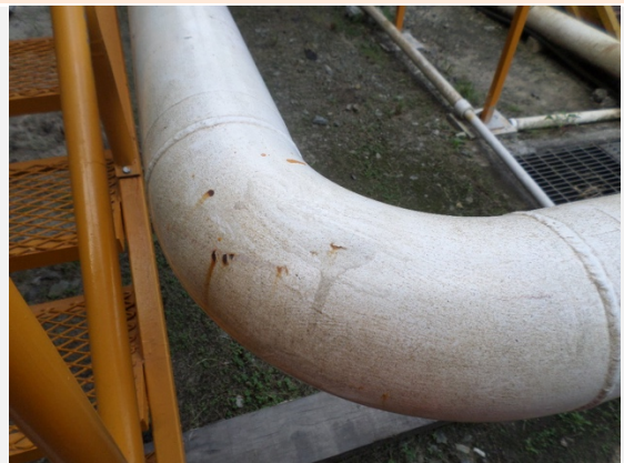
Photo: 16 Comment: Isolated coating damage and surface corroded spots, at elbow, location no 68
