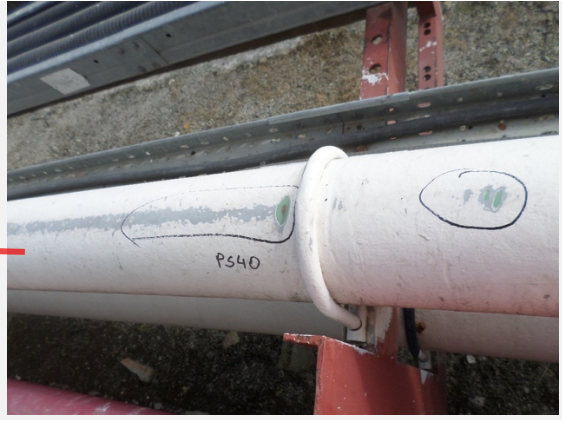
Photo: 32 Comment: Isolated minor coating breakdowns on the line, location: around pipe support PS40
