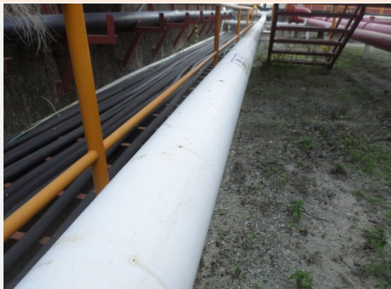
Photo: 24 Comment: Isolated minor coating breakdowns on the line, location: between pipe supports PS35 and PS36
