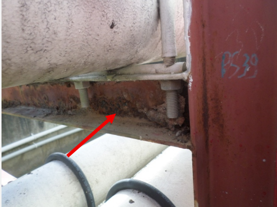
Photo: 7 Comment: Coating breakdown and surface corrosion at the U-beam at support PS39
