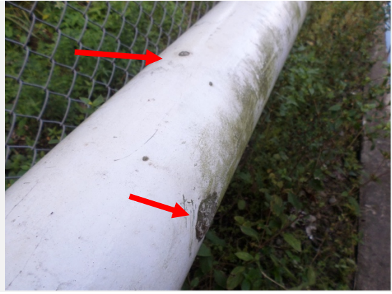
Photo: 8 Comment: Isolated concrete spatter noted at the line, location: between pipe supports PS6 and PS7
