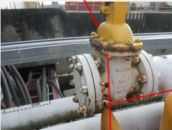
Photo: 27 Comment: General view of the Gate Valve, corrosion noted at the body and the flange fasteners. Valve upstream of T-Piece.
