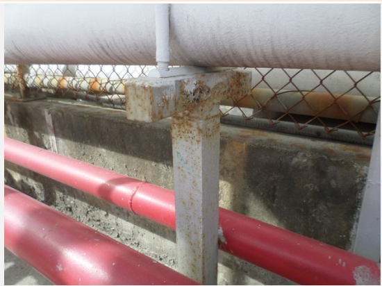
Photo: 9 Comment: PS55 – Coating breakdown and surface corrosion on the beam support
