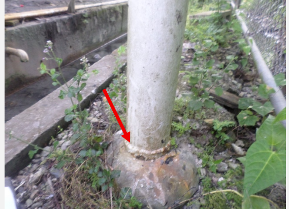
Photo: 2 Comment: Pipe support foundation, at PS7 found with surface corrosion at the foundation.
