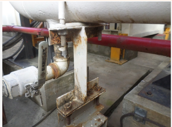
Photo: 18 Comment: PS60 - Coating breakdown and surface corrosion on the support
