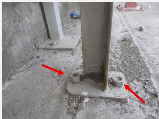
Photo: 11 Comment: PS55 – Insufficient thread engagement at the fasteners, at the base of the support
