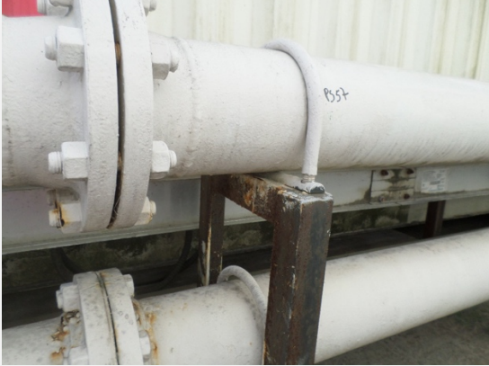
Photo: 13 Comment: PS57 - Coating breakdown and surface corrosion on the beam support
