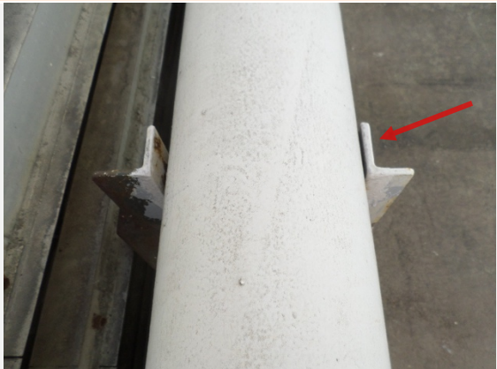
Photo: 36 Comment: Direct contact, "metal to metal", between pipe and the guide, at Pipe support PS58
