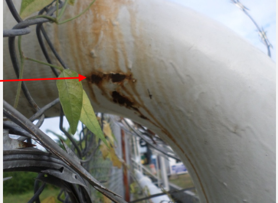
Photo:2 Comment: Elbow component, location 5 on iso, found with localized corrosion
