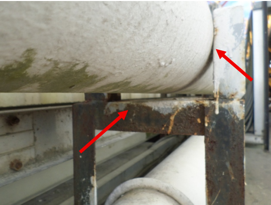
Photo: 15 Comment: PS58 – Direct contact, “metal to metal”, between pipe and the guide, air gap of 12mm between the pipe and the support. Coating damage and surface corrosion noted on the guide support
