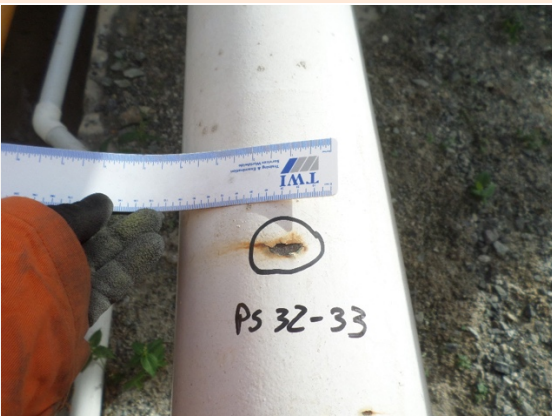
Photo: 23 Comment: Localized corrosion spot (30mm long), surface corrosion at 12 o'clock, location: between pipe supports PS32 and PS33
