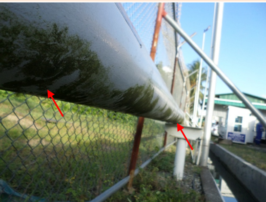
Photo:5 Comment: Algae present at the 6 o'clock location, typical to the entire line.
