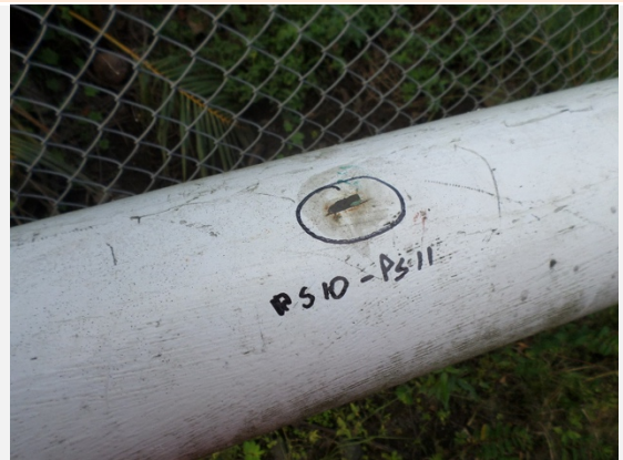
Photo: 10 Comment: Localized corrosion spot (Dia 30mm), surface corrosion at 12 o'clock, location: between pipe supports PS10 and PS11
