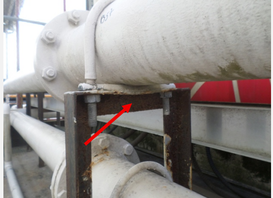
Photo: 14 Comment: L-profile beam PS57 found with localized surface corrosion at inner side of beam and found bent, No change in condition since last inspection
