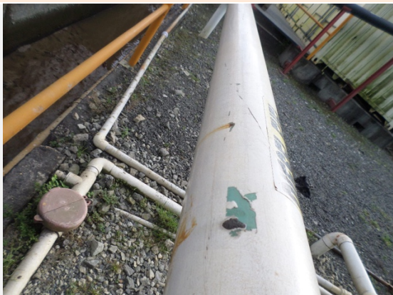
Photo: 21 Comment: Coating damage and concrete spatter noted at the line, location: between pipe supports PS28 and PS29
