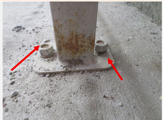
Photo: 12 Comment: PS56 – Insufficient thread engagement and the air gap between the nut and the joint surface, at the base of the support
