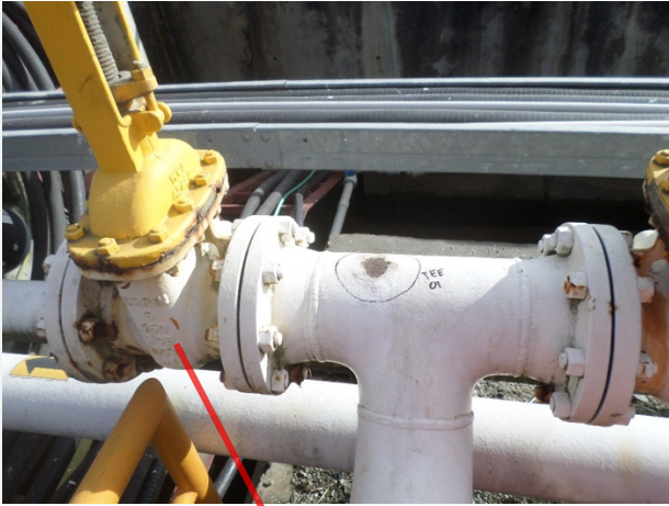
Photo: 25 Comment: Localized corrosion spot (Dia 65mm), surface corrosion at 12 o'clock, location: T-piece, at location 105
