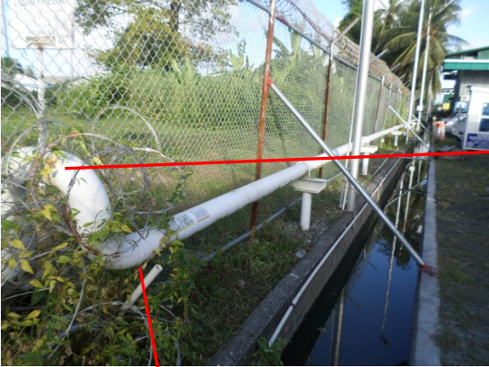
Photo: 1 Comment: View of the start of the Fuel Diesel line (Sol to Gysbi)
