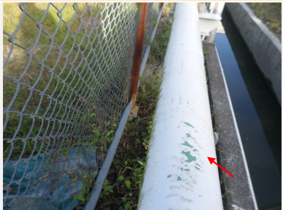
Photo:6 Comment: Topcoat damage to the section of the line, upstream of Pipe support PS1.
