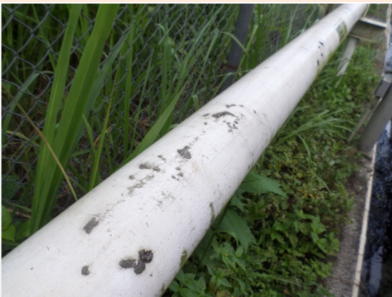
Photo: 15 Comment: Isolated concrete spatter noted at the line, location: between pipe supports PS12 and PS13
