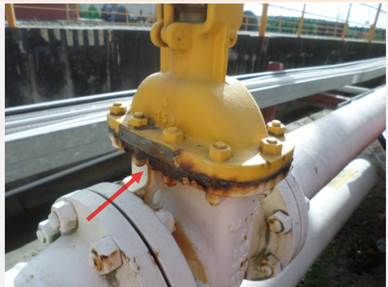
Photo: 30 Comment: Crevice corrosion noted on the bonnet to body, flanged joint. Valve downstream of T-Piece.
