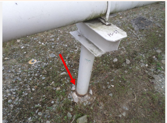
Photo: 4 Comment: Pipe support foundation, at PS19 found with corrosion at the foundation.
