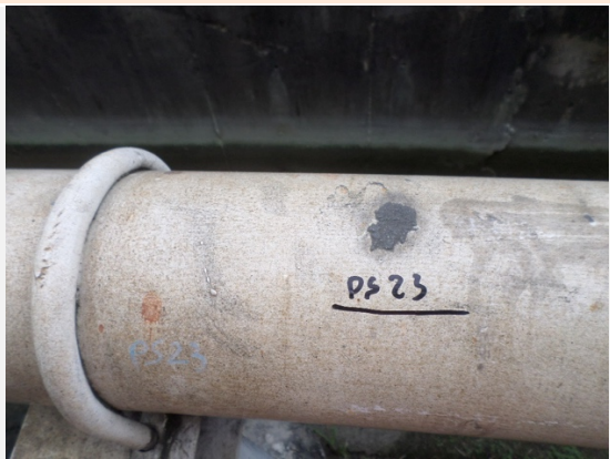
Photo: 17 Comment: Isolated concrete spatter noted at the line, location: downstream of pipe supports PS23
