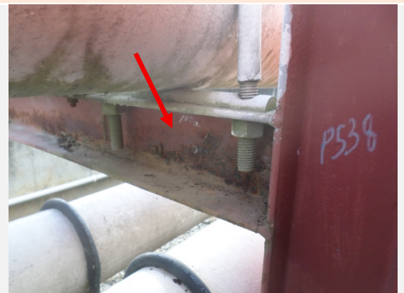
Photo: 6 Comment: Coating breakdown and surface corrosion at the U-beam at support PS38
