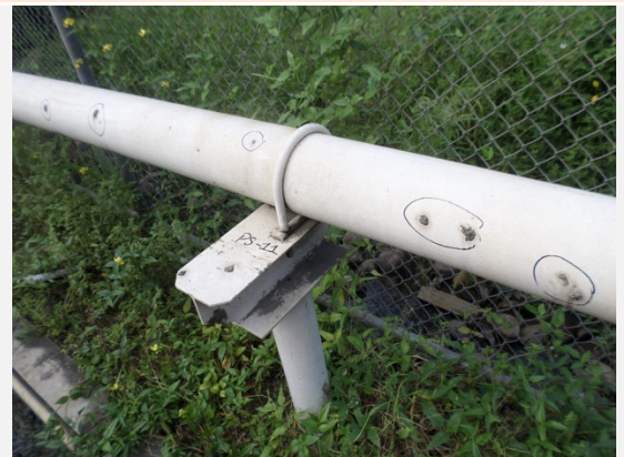
Photo: 12 Comment: Localized concrete spatter located downstream and upstream of pipe support PS11.
