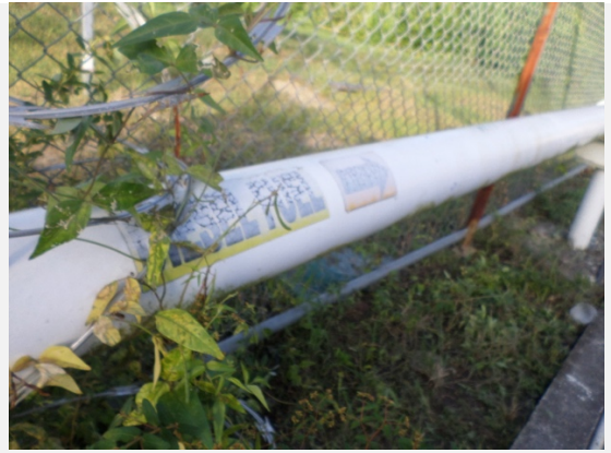
Photo:4 Comment: Faded stickers (due to UV) at the beginning of the line
