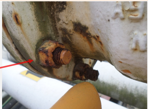
Photo: 28 Comment: Close-up photo - Surface corrosion noted on the flange fasteners. Valve upstream of T-Piece.
