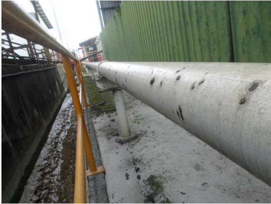
Photo: 19 Comment: Isolated concrete spatter noted at the line, location: between pipe supports PS26 and PS27
