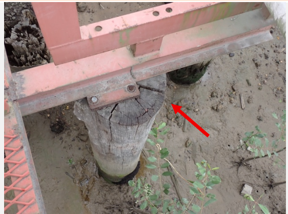
Photo: 22 Comment: PS45 – Wooden pillar -A, with significant cracking along the top grain visible, some oxidation and rust visible on the fasteners.
