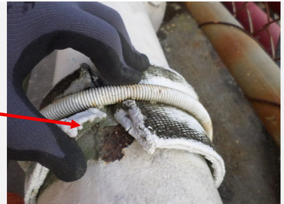
Photo: 4 Comment: PS3 – evidence of coating breakdown and corrosion evident under the fabric.
