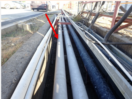
Photo: 5 Comment: Area of the line from PS18 to PS24, where the supports are positioned in the water. No access to the base of the supports, possible corrosion under the water level.
