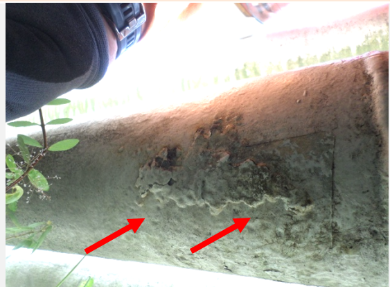
Photo: 10 Comment: Isolated, corrosion blister at 6 o'clock, located at points 33&34 on ISO
