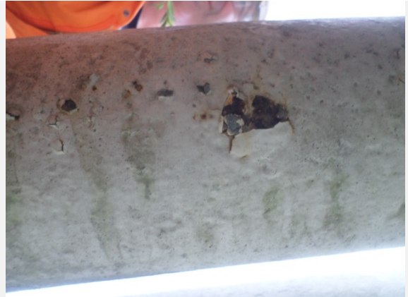
Photo: 8 Comment: Isolated, corrosion blister at 6 o'clock, location: at point 32, between supports PS4 and PS5
