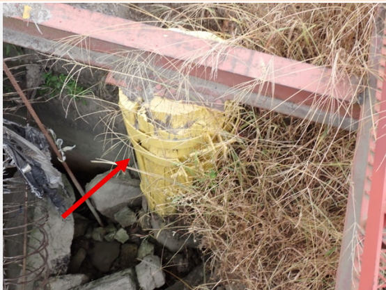
Photo: 21 Comment: PS44 – Wooden pillar, braced with metal clamps, visible cracks
