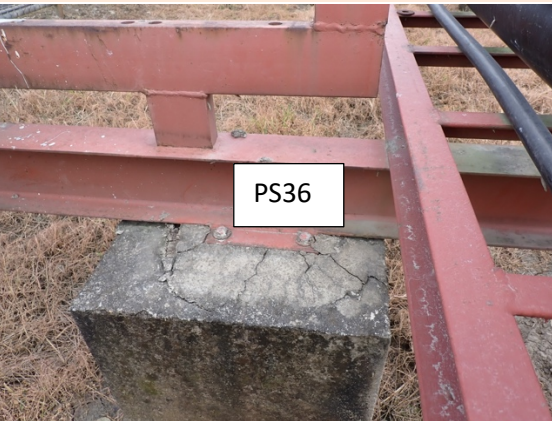
Photo: 17 Comment: PS36 – Concrete foundation, cracks around the base plate
