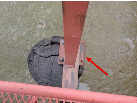
Photo: 29 Comment: PS48 – Wooden pillar - A, with significant cracking along the top grain visible. The bracket not centered over the pillar -missing two, out of 4 fixing bolts
