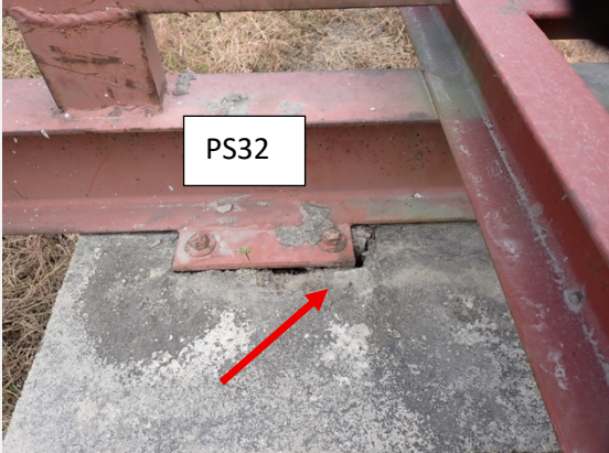
Photo: 13 Comment: PS32 – Concrete foundation, damaged, hollow space under the base plate
