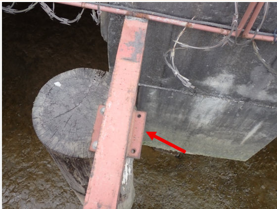
Photo: 30 Comment: PS48 – Wooden pillar - B. The bracket not centered over the pillar -missing two, out of 4 fixing bolts
