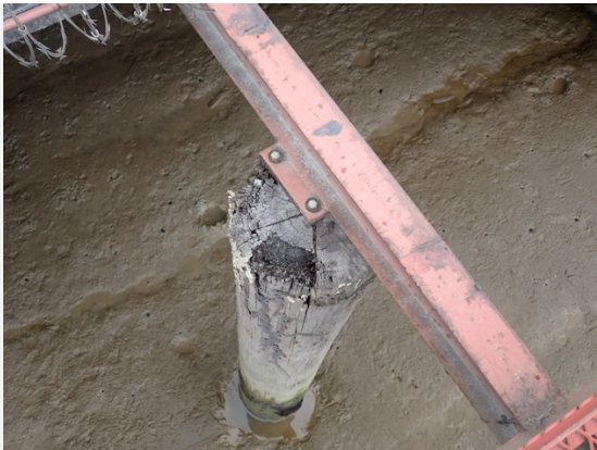
Photo: 25 Comment: PS46 – Wooden pillar - B, with significant cracking along the top grain visible.
