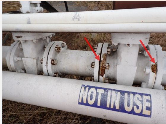
Photo: 27 Comment: coating damage and surface corrosion on the valve flange, some rusting on the fasteners. Location: point 171
