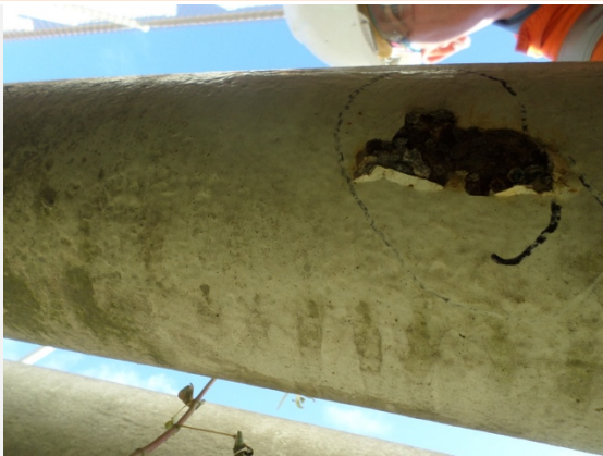
Photo: 15 Comment: Isolated, corrosion blister at 6 o'clock, location: at point 41, between supports PS8 and PS9
