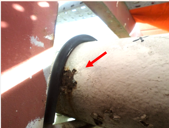
Photo: 9 Comment: Isolated coating damage with surface corrosion, located at 9 o'clock, at PS5
