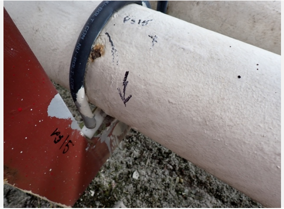
Photo: 20 Comment: Isolated coating damage with surface corrosion at 11 o'clock, location: at support PS15
