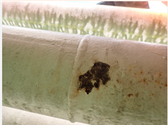
Photo: 17 Comment: Isolated coating damage with surface corrosion, located at 6 o'clock, at P45,46, between PS10 and PS11
