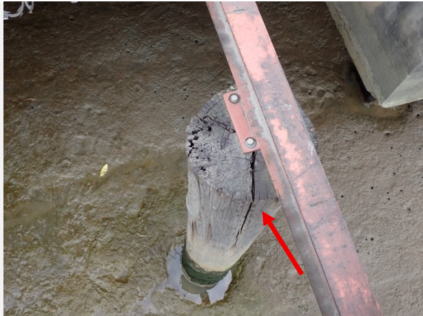
Photo: 28 Comment: PS47 – Wooden pillar - B, with significant cracking along the top grain visible
