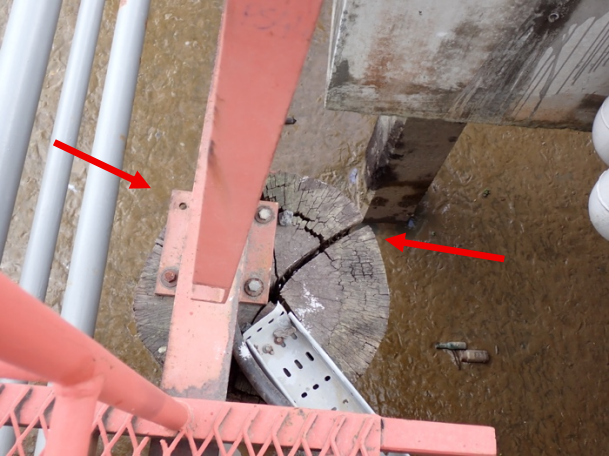
Photo: 31 Comment: PS49 – Wooden pillar - A, with significant cracking along the top grain visible. The bracket not centered over the pillar -missing one, out of 4 fixing bolts
