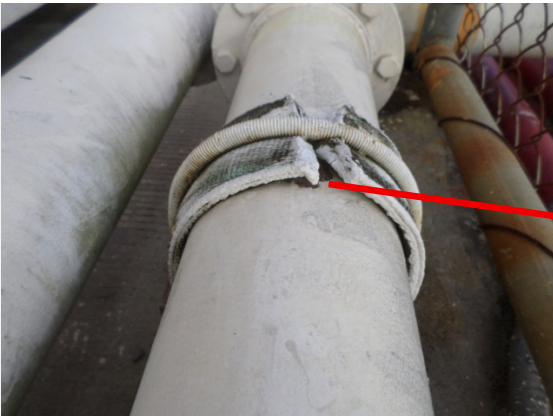
Photo: 3 Comment: Pipe support PS3- Random fabric used as U-bolt sleeve, possible corrosion under the fabric. To be replaced with I-Rod system
