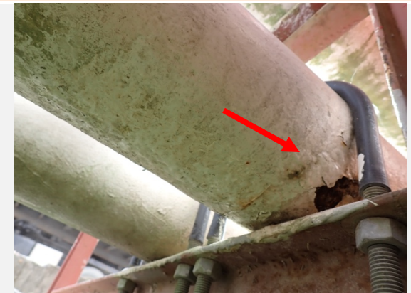
Photo: 18 Comment: Crevice corrosion present at piping, at 6 o'clock location, at pipe support PS 10.
