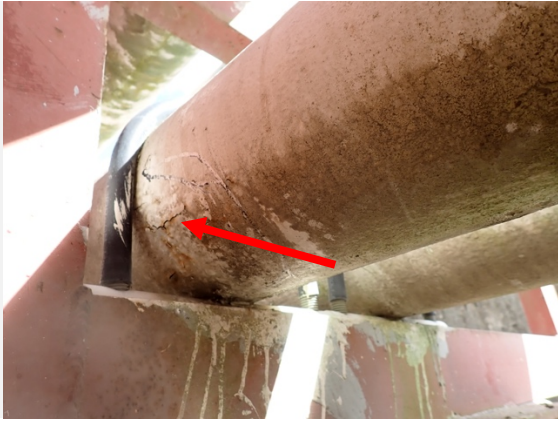
Photo: 19 Comment: Isolated, corrosion blister at 7 o'clock, location: at support PS12
