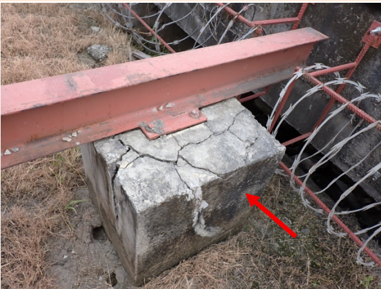
Photo: 16 Comment: PS35 – severe damage to the concrete foundation - B. Repair required
