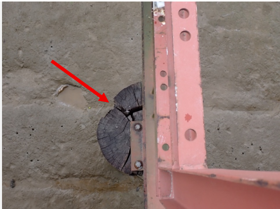
Photo: 26 Comment: PS46 – Wooden pillar - A, with significant cracking along the top grain visible. The bracket not centered over the pillar -missing one, out of 4 fixing bolts
