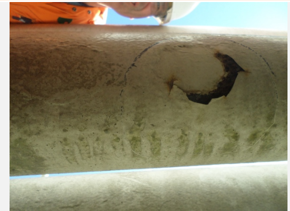
Photo: 16 Comment: Isolated, corrosion blister at 6 o'clock, location: at point 44, between supports PS9 and PS10
