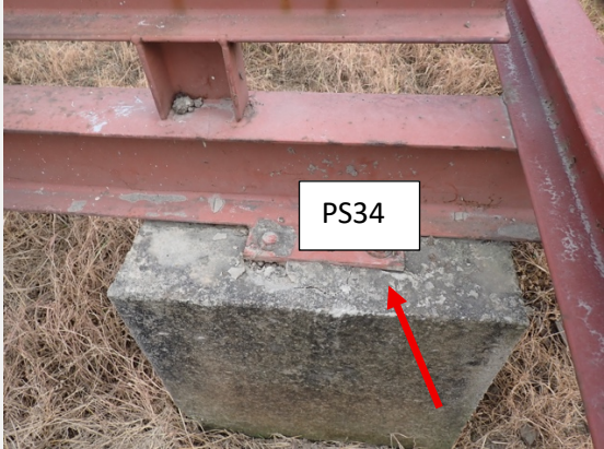
Photo: 14 Comment: PS34 – Concrete foundation, cracks around the base plate
