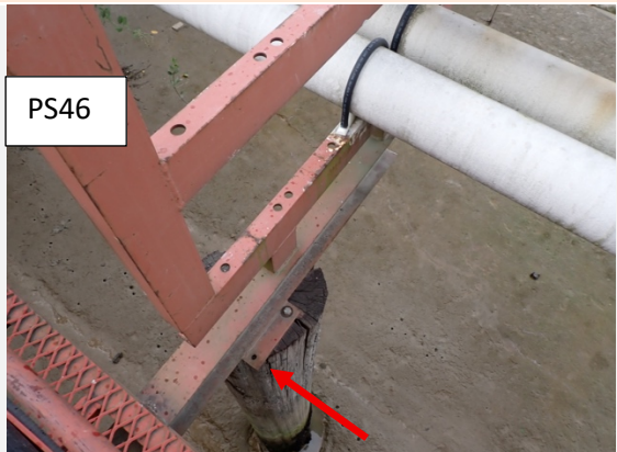
Photo: 24 Comment: PS46 – The bracket not centered over the pillar A-missing one, out of 4 fixing bolts
