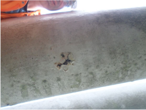
Photo: 7 Comment: Isolated, corrosion blister at 6 o'clock, location: at point 32, between supports PS4 and PS5
