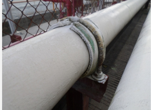
Photo: 2 Comment: Pipe support PS2- Random fabric used as U-bolt sleeve, possible corrosion under the fabric. To be replaced with I-Rod system
