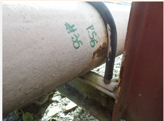
Photo: 12 Comment: Isolated coating damage with surface corrosion, located at 9 o'clock, at PS6
