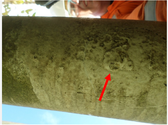
Photo: 14 Comment: Isolated, corrosion blister at 6 o'clock, location: at point 41, between supports PS8 and PS9
