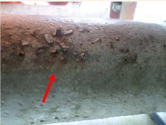
Photo: 11 Comment: Isolated, corrosion blister at 6 o'clock, located at points 33&34 on ISO
