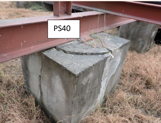
Photo: 18 Comment: PS40 – severe damage to the concrete foundation. Repair required
