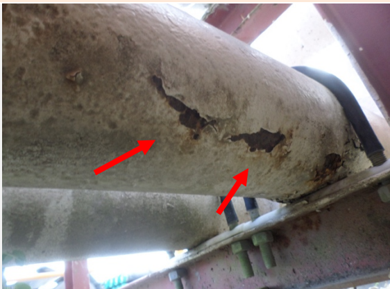
Photo:6 Comment: Isolated coating damage with surface corrosion, located at 7 o'clock, location: downstream of PS4
