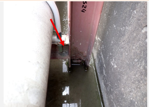
Photo: 6 Comment: Pipe support PS24, base covered by standing water, surface corrosion present at the base.
