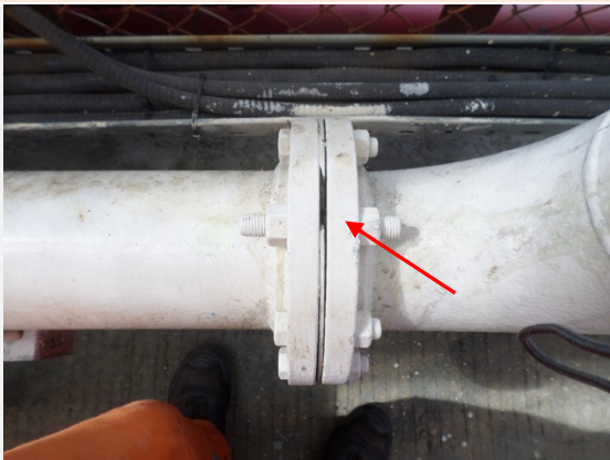
Photo:3 Comment: Damaged flange gasket at 12 o'clock. Second flange on the line, point no 12 on ISO. No leak present. Reported to the Fuel Pump skid supervisor.
