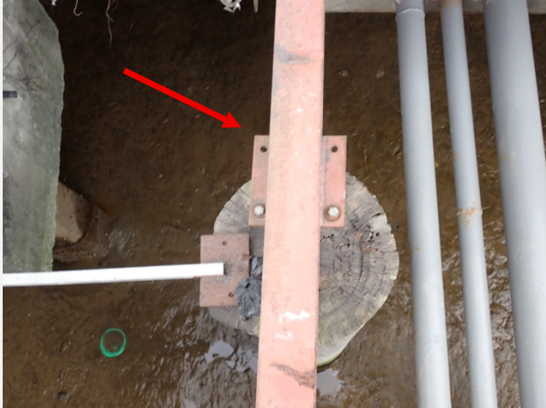
Photo: 32 Comment: PS49 – Wooden pillar - B. The bracket not centered over the pillar -missing two, out of 4 fixing bolts
