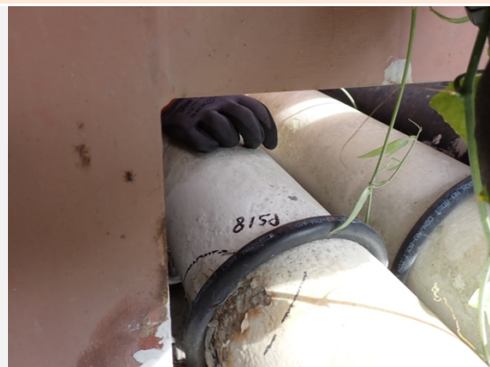
Photo: 23 Comment: Isolated, corrosion blister at 10 o'clock, location: at support PS18
