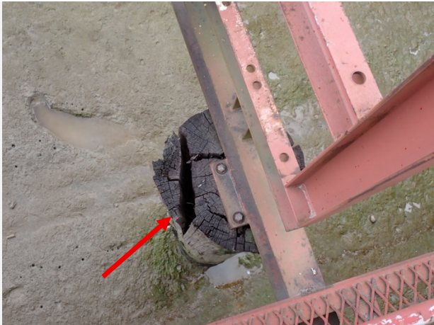
Photo: 27 Comment: PS47 – Wooden pillar - A, with significant cracking along the top grain visible
