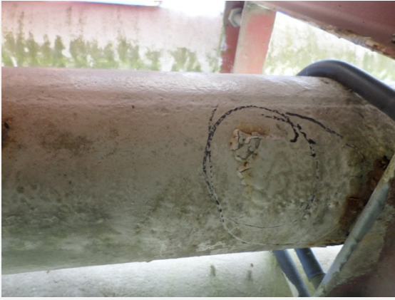
Photo: 13 Comment: Isolated, corrosion blister at 6 o'clock, location: at pipe support PS8.
