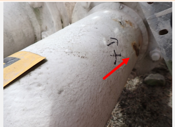
Photo: 22 Comment: Isolated coating damage with surface corrosion, located at 9 o'clock, at P78, downstream of flange, between PS17 and PS18
