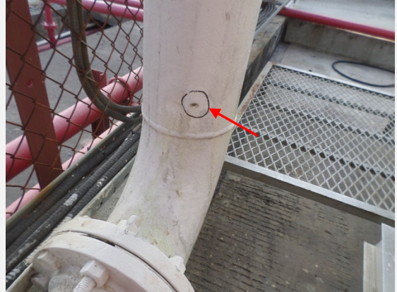
Photo:2 Comment: Isolated coating damage to the line, location no.9 on ISO
