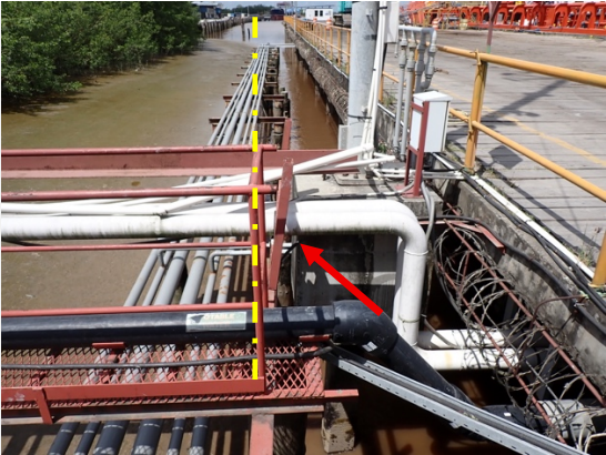
Photo: 33 Comment: PS49 – support frame bend to the side
