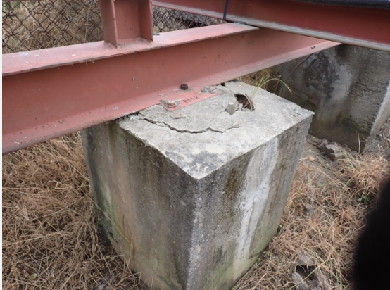
Photo: 19 Comment: PS43 – Concrete foundation, cracks around the base plate
