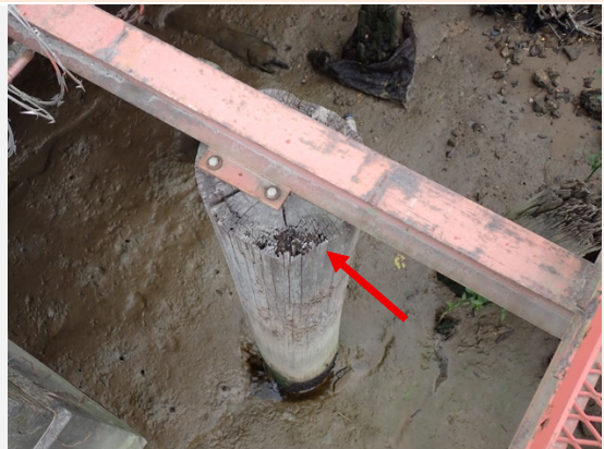
Photo: 23 Comment: PS45 - Wooden pillar - B, with significant cracking along the top grain visible
