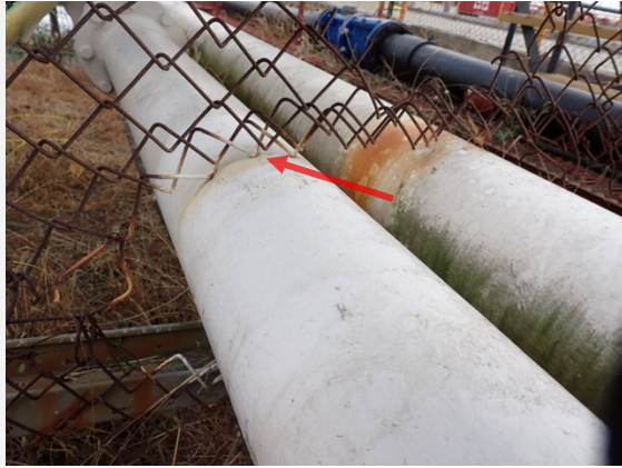
Photo: 26 Comment: Metal-to-metal contact with the fence, location: downstream of pipe support PS43
