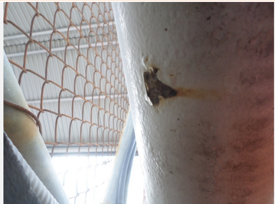
Photo:4 Comment: Isolated coating damage with surface corrosion 30mm Dia, located at 5 o'clock, location: between pipe supports PS1 and PS12
