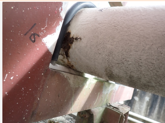
Photo: 21 Comment: Isolated coating damage with surface corrosion at 9 o'clock, location: at support PS16
