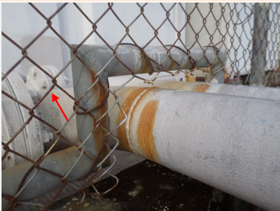
Photo:5 Comment: Staining, from the metal fencing, noted at the location no 23. No damage to coating noted yet.
