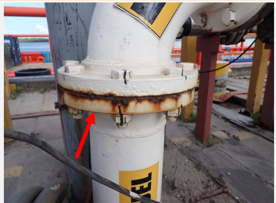
Photo: 10 Comment: Berth 2 Manifold. Crevice corrosion at the flange, at point 2.
