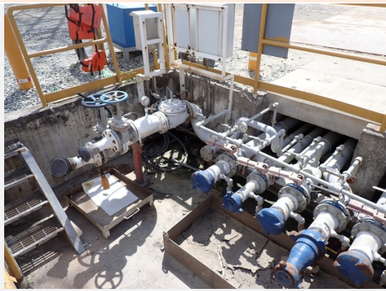
Photo: 48 Comment: Berth 4. General view of the manifold 4.
