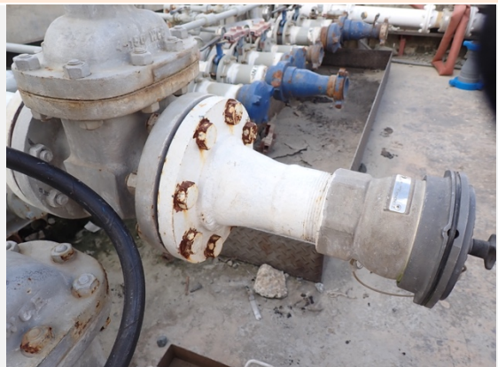
Photo: 52 Comment: Berth 4. Surface corrosion around and at the fasteners at the termination spool at point 186
