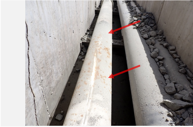
Photo: 43 Comment: Berth 4, scattered rusting points at line, location point 123.
