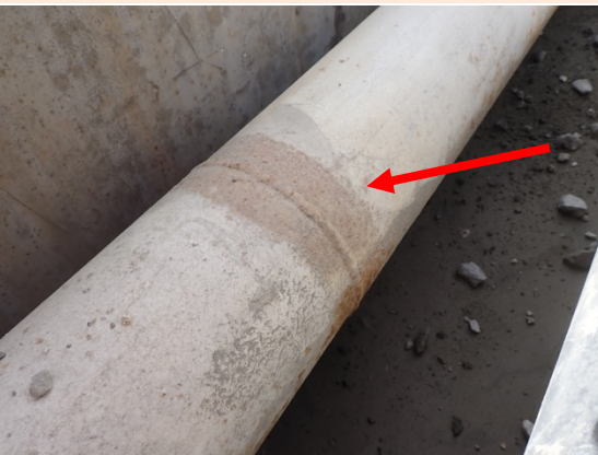
Photo: 23 Comment: Berth 3. Surface corrosion noted around weld, at point 20,21. Previously removed coating around the weld, was not re-applied.
