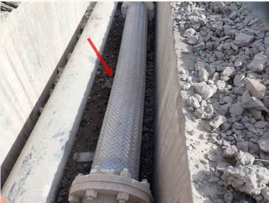
Photo: 27 Comment: Berth 3. A flexible, SS metal braided spool, installed on the line, at position 28-29. Found in good condition.
