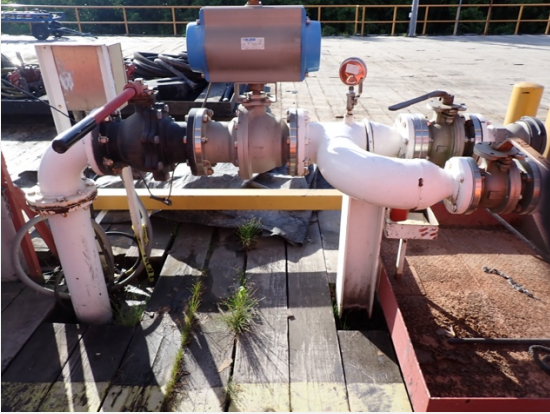
Photo: 1 Comment: Berth 1 Manifold. General view.
