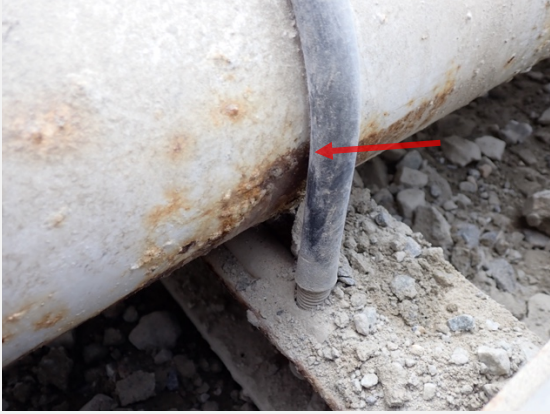
Photo: 25 Comment: Berth 3. Isolated spot with coating damage and surface corrosion, at pipe support, PS7
