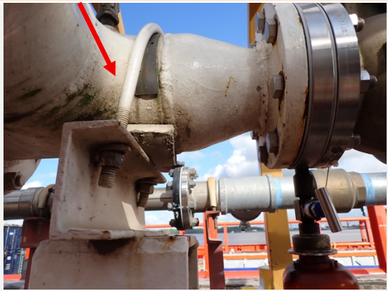
Photo: 5 Comment: Berth 2 Manifold – U-bolt misaligned due to the geometric constraints of the T-piece.
