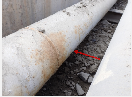
Photo: 26 Comment: Berth 3. Rusting spots at weld, point 26, 27
