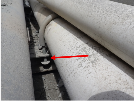
Photo: 13 Comment: Berth 4. Fastener (nut) not done up, possible thread damage. PS32, typical to all supports, between PS 24 to PS34
