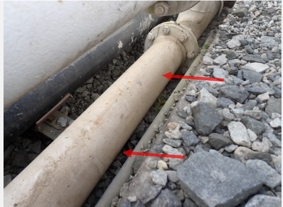
Photo: 32 Comment: Berth 3, Minor, mechanical coating damage areas (paint chips). Spool, between points 77 and 79.
