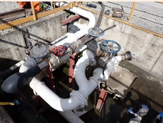
Photo: 29 Comment: Berth 3. General view of the manifold 3.
