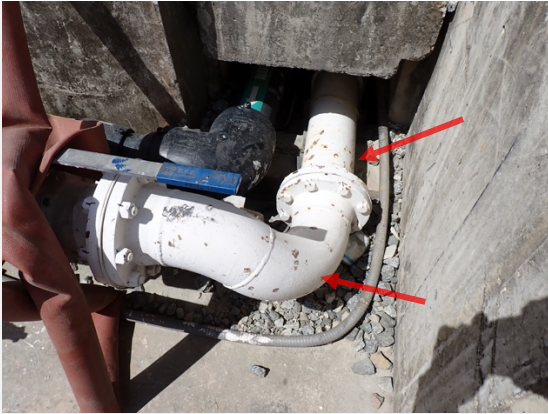
Photo: 49 Comment: Berth 4. Scattered coating damage noted at location between points 150 and 157.
