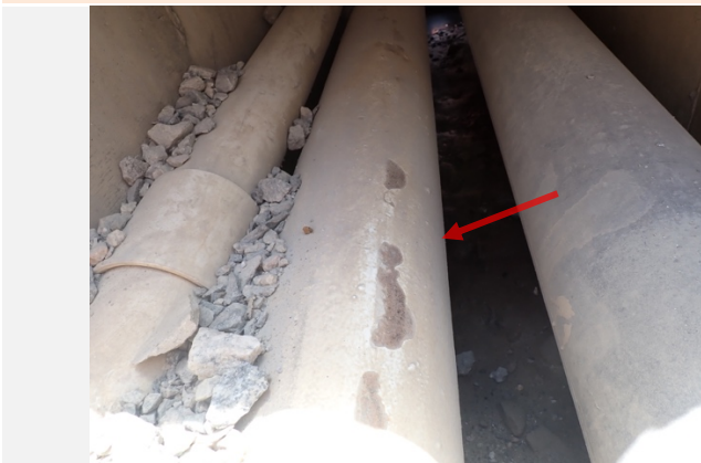
Photo: 47 Comment: Berth 4. Coating damage noted at 12 o'clock location at position 147.
