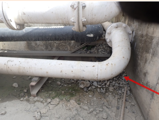
Photo: 33 Comment: Berth 3, Minor, mechanical coating damage areas (paint chips). Spool, between points 80 and 89.
