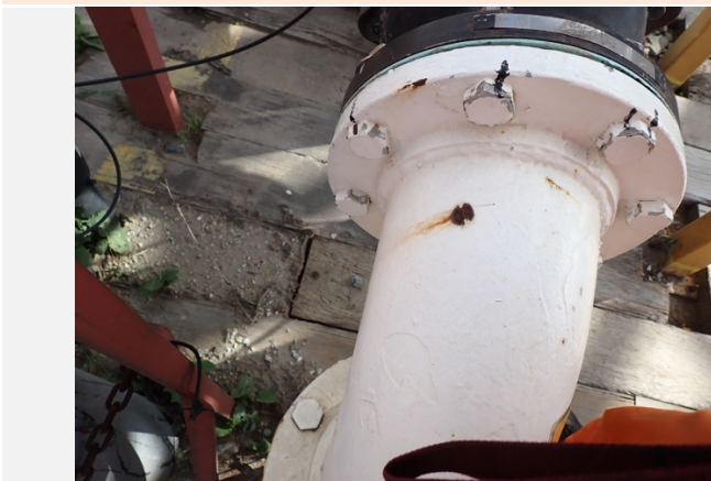
Photo: 11 Comment: Berth 2 Manifold. Isolated coating damage area at elbow extrados, at point 4.
