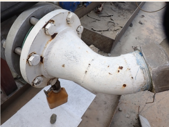
Photo: 53 Comment: Berth 4. Isolated coating damages at the termination spool at point 190.
