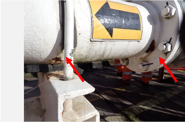
Photo: 7 Comment: Berth 1 Manifold, isolated coating damage and surface corrosion at the weld at point 6 & 8.
