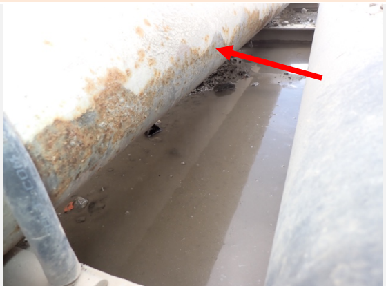
Photo: 22 Comment: Berth 3. General view, topcoat missing at the bottom half, along the line at the berth 3, upstream of manifold. Surface corrosion noted.
