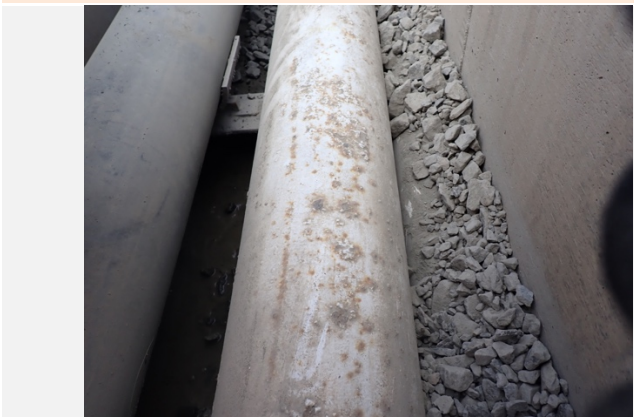
Photo: 45 Comment: Berth 4. Scattered corrosion blisters note at 12 o'clock location at line, point 144.
