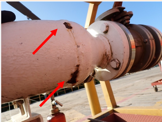
Photo:5 Comment: Berth 1 Manifold, isolated coating damage and surface corrosion at the weld at point 12.
