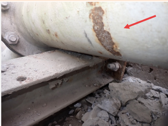
Photo: 35 Comment: Berth 3. Coating damage and surface corrosion, noted at 4 o'clock location at support area, PS20
