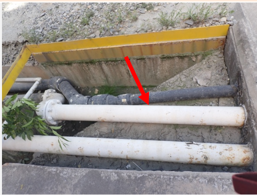
Photo: 15 Comment: Berth 3. General view of the Fuel line at the penetration, between berth 2 and berth 3.
