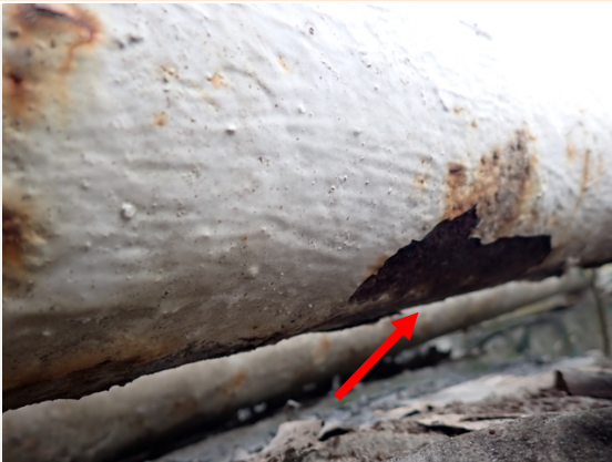
Photo: 17 Comment: Berth 3. Isolated coating damage and surface corrosion, located at 6 o'clock position at point 4.
