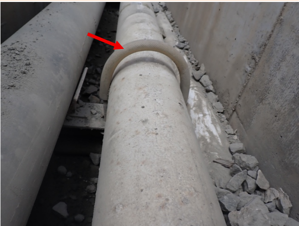
Photo: 11 Comment: Misaligned U-bolt with airgap present, between top side of the pipe and the U-bolt. Pipe support PS32
