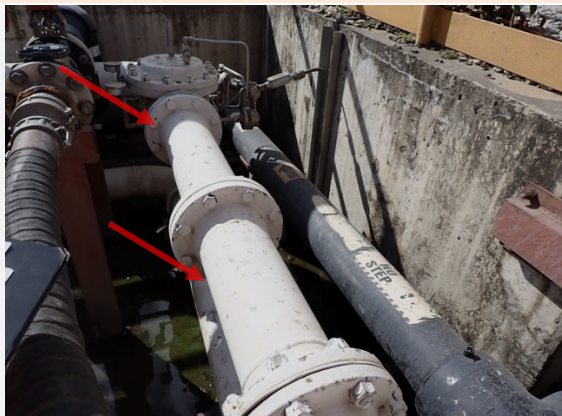
Photo: 30 Comment: Berth 3. Minor, mechanical coating damage areas (paint chips). Spools, between points 47 and 53.
