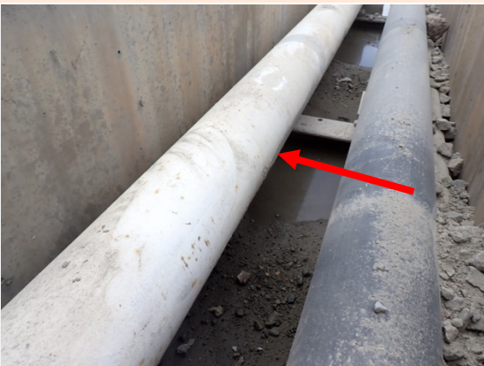
Photo: 21 Comment: Berth 3. General view, scattered minor rust spots along the entire line.
