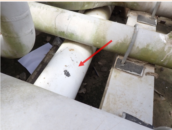
Photo: 51 Comment: Berth 4. Isolated coating damages at the line at point 170
