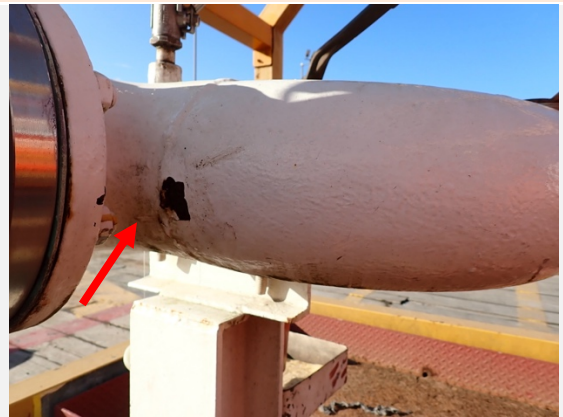
Photo:4 Comment: Berth 1 Manifold, isolated coating damage and surface corrosion at the weld at point 10.
