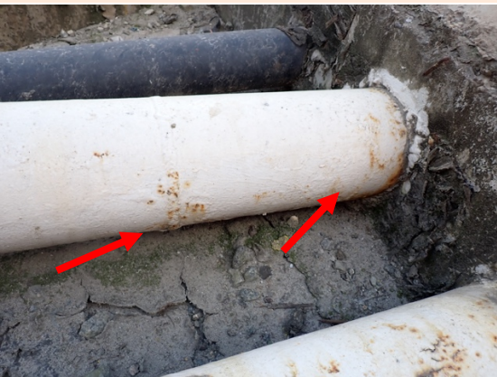
Photo: 16 Comment: Berth 3. Minor surface corrosion rust spots noted at the line, at the point 1.
