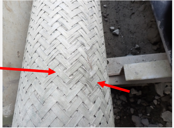
Photo: 20 Comment: isolated, minor ss braid damage, noted at 12 o'clock.
