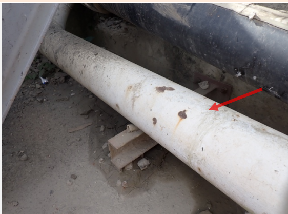
Photo: 34 Comment: Berth 3, Scattered coating damage areas, with surface corrosion, at point 100.
