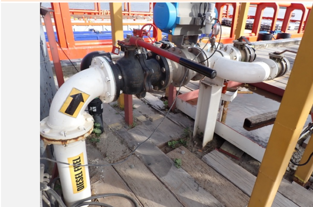
Photo: 9 Comment: Berth 2 Manifold. General view.
