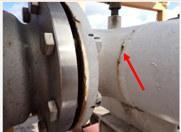
Photo: 12 Comment: Berth 2 Manifold, SS bolts used without any insulation on the carbon steel flange. Danger of galvanic corrosion. Surface corrosion noted at weld at point 10.
