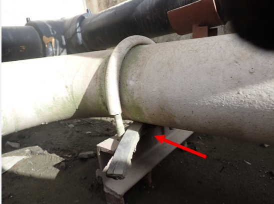
Photo: 8 Comment: Berth 3. Shim at PS15 not aligned with the support's base.
