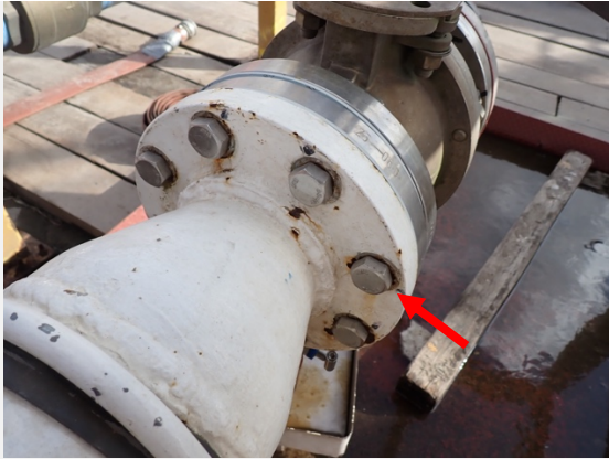
Photo: 13 Comment: Comment: Berth 2 Manifold, SS bolts used without any insulation on the carbon steel flange.
