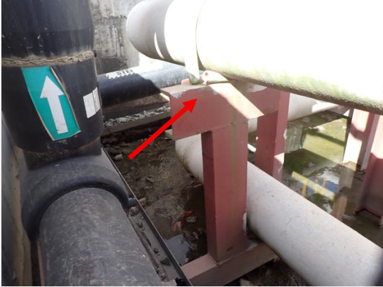
Photo: 7 Comment: Berth 3 manifold, an elastic rubber tubing used as a shim, PS11, typical occurrence to most of the supports on the line.
