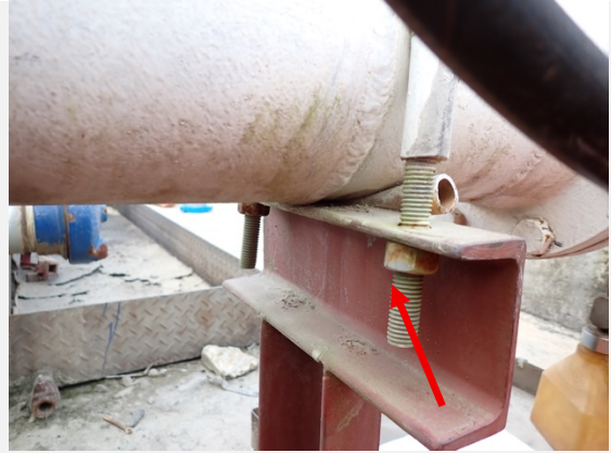
Photo: 14 Comment: Berth 4. Damaged shim and metal-to-metal contact between pipe and support at PS39
