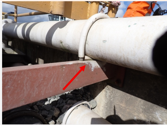
Photo: 6 Comment: Berth 3 manifold, an elastic rubber tubing used as a shim, typical occurrence to most of the supports on the line.
