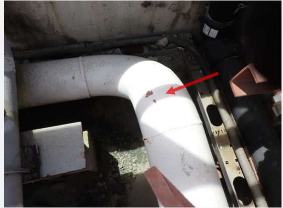
Photo: 50 Comment: Berth 4, isolated coating damage at elbow at point 165
