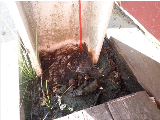
Photo: 3 Comment: Berth 1 Manifold. Coating damage and the corrosion at the support base.
