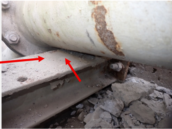
Photo: 10 Comment: Berth 3. Missing shim and metal-to-metal contact between pipe and support at PS20
