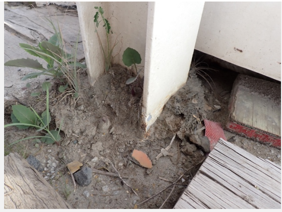
Photo: 4 Comment: Berth 2 Manifold, the support base covered by soil, coating damage and surface corrosion likely.
