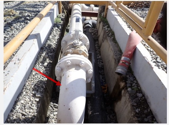
Photo: 28 Comment: Berth 3. Minor, mechanical coating damage areas (paint chips). Elbow, point 38.
