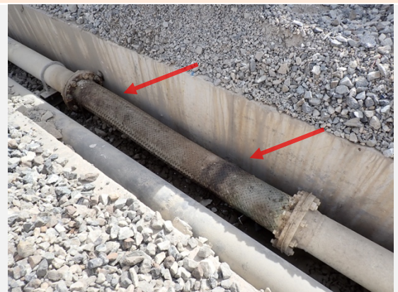
Photo: 36 Comment: Evidence of seep/leak was noted at the 5ft long, flexible, metal braided spool, position between points 109 and 110
