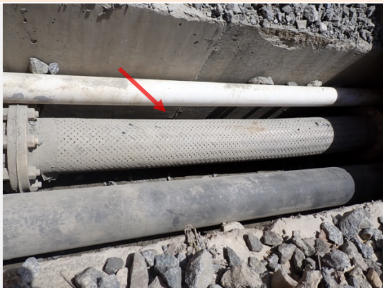
Photo: 46 Comment: Berth 4. A flexible, SS metal braided spool, installed on the line, at position 148-149. Found in good condition.
