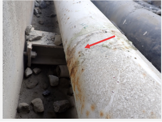
Photo: 44 Comment: Berth 4. Isolated coating damage and rusting spots noted at 9 o'clock location at weld point 130, 131
