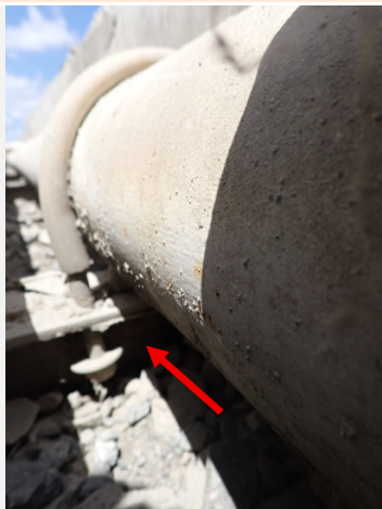
Photo: 12 Comment: Berth 4. Fastener (nut) not done up, possible thread damage. PS31, typical to all supports, between PS 24 to PS34
