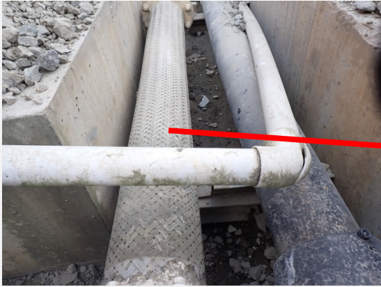
Photo: 19 Comment: Berth 3. A flexible, SS metal braided spool, installed on the line, at position 14-15. Found in generally good condition.
