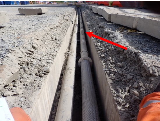
Photo: 18 Comment: Berth 3. General view of the line installed inside the utilidor, with covers lifted.
