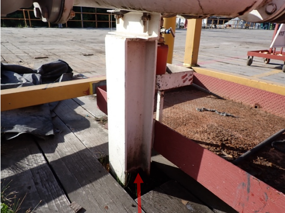
Photo: 1 Comment: Berth 1 Manifold. PS1 General view of the support at TEE-Piece
