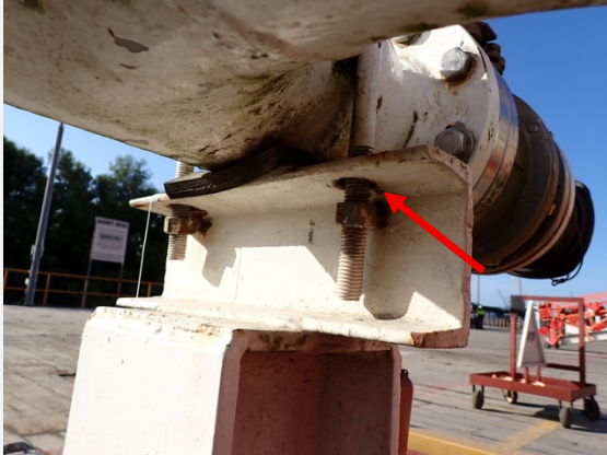
Photo: 2 Comment: Berth 1 Manifold. Fastener (nut) not done up, possible thread damage.
