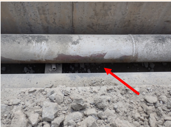
Photo: 24 Comment: Berth 3. General view, topcoat missing at the bottom half, along the line at the berth 3, upstream of manifold
