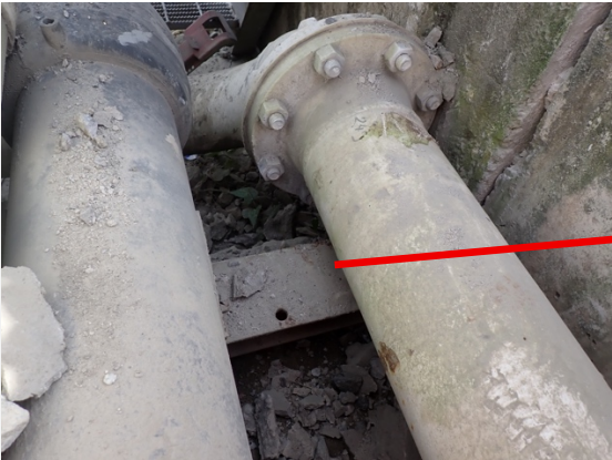
Photo: 9 Comment: Berth 3. Missing shim and metal-to-metal contact between pipe and support at PS20
