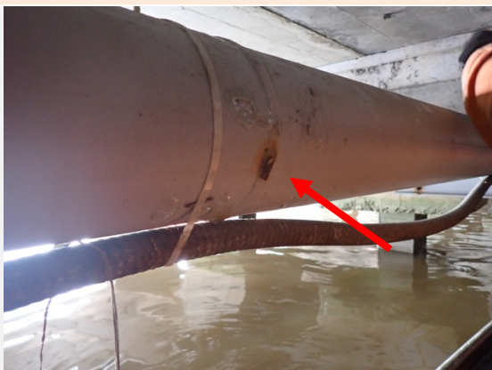
Photo: 11 Comment: Isolated coating damage and surface corrosion noted on the weld, at point 261, 262.
