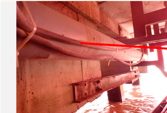
Photo: 17 Comment: Heavily corroded section of the line, just below the penetration at the manifold, at Berth 2. Multiple areas with corrosion blisters present, location: between point 292 and 299
