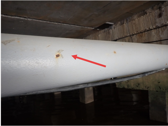
Photo: 26 Comment: isolated coating damage, at point 316
