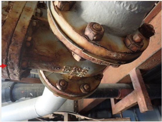
Photo: 28 Comment: Isolation valve, for the manifold at berth 3, heavy corrosion present on the body and fasteners, location points 347 and 348.
