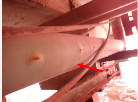
Photo: 20 Comment: Heavily corroded section of the line, just below the penetration at the manifold, at Berth 2. Multiple areas with corrosion blisters present, location: point 293
