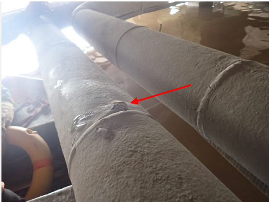
Photo:3 Comment: Isolated corrosion and minor scale present at 12 o'clock position, at the weld at location 201,202
