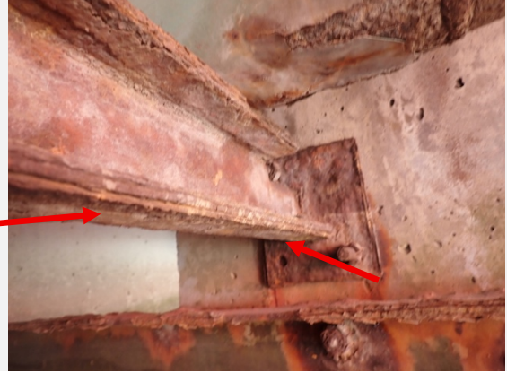
Photo: 8 Comment: Heavily corroded support, PS74 with scale present on the entire support structure. Located just below the penetration to the manifold area, at Berth 2.
