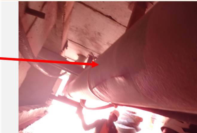
Photo: 18 Comment: Heavily corroded section of the line, just below the penetration at the manifold, at Berth 2. Multiple areas with corrosion blisters present, location: point 293.
