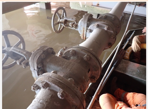
Photo: 12 Comment: Two isolation valves, at point 264, surface corrosion on the bodies and heavy corrosion noted on the fasteners
