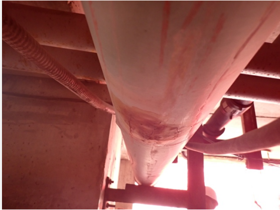
Photo: 19 Comment: Heavily corroded section of the line, just below the penetration at the manifold, at Berth 2. Multiple areas with corrosion blisters present, location: point 293
