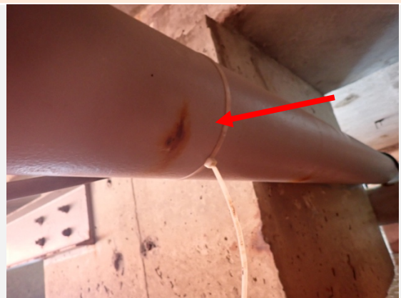
Photo: 23 Comment: Isolated coating damage and surface corrosion noted on the line, at point 310.
