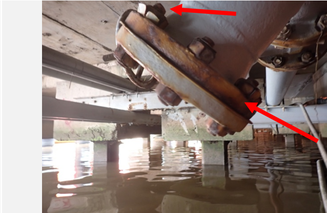
Photo: 14 Comment: Crevice corrosion and fasteners' corrosion at the blind, installed between two valves.
