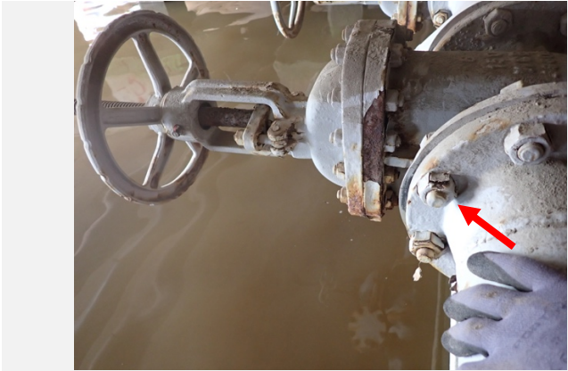
Photo: 13 Comment: Two isolation valves, at point 264, surface corrosion on the bodies and heavy corrosion noted on the fasteners
