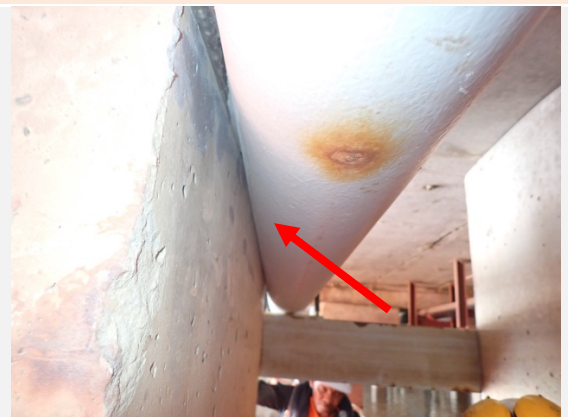
Photo: 24 Comment: Direct contact, between the line and the concrete wall, at point 310
