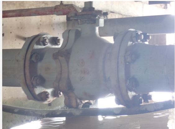
Photo:4 Comment: Valve, located between points 213 and 214. Corroded body and flange fasteners
