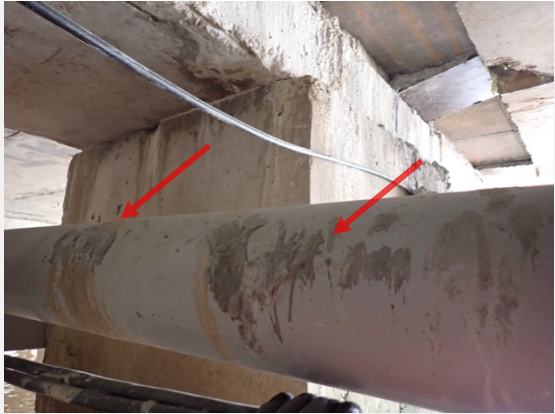
Photo: 25 Comment: Thick - external, like-concrete, deposits noted at 2 o'clock location, at point 316.
