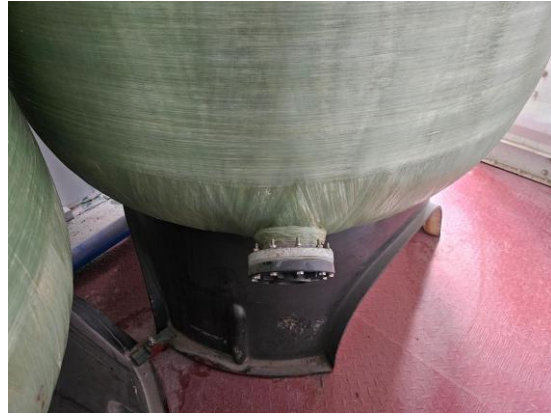
Photo M-04 - Typical lower vessel connection and support arrangement.
