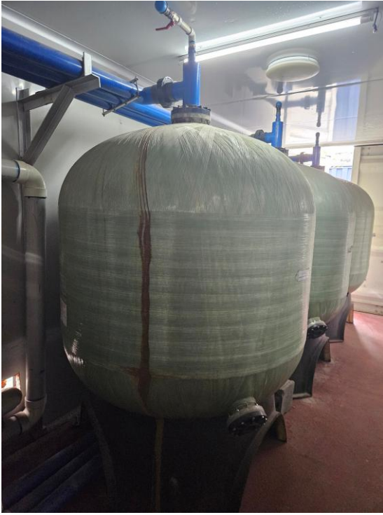
Photo M-07 - General view of pressure vessels and upper piping within the container.
