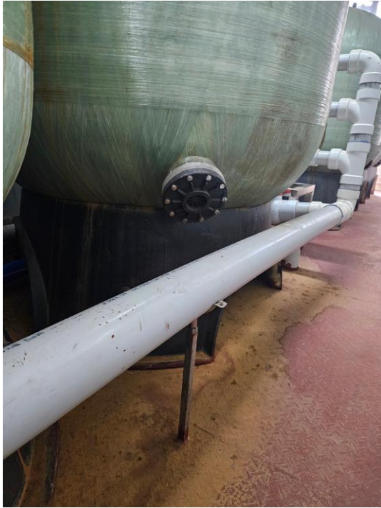
Photo M-01 - Typical lower vessel connection with foreground drain/header piping.
