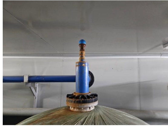
Photo M-06 - Upper vessel connection and top piping arrangement.
