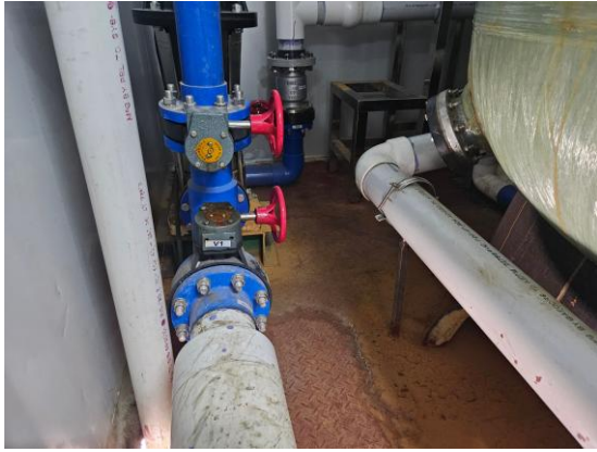
Photo M-03 - Valve and piping arrangement at the end of the filter line.
