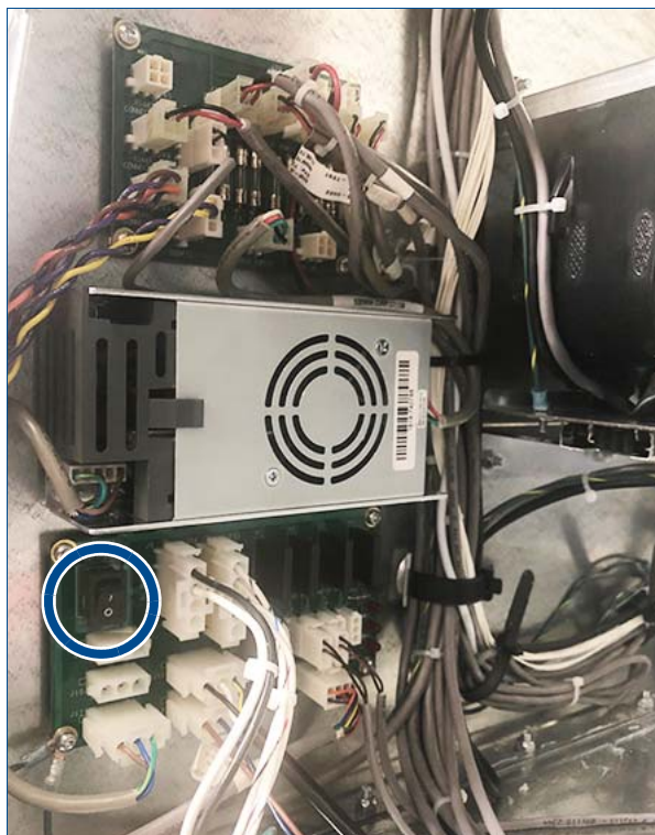
Figure 5-1 Dispenser ON/OFF Switch on A/C Power Distribution Board
